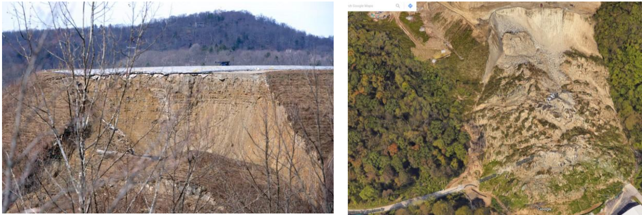
Figure 2. The failure of Yeager airport expansion runway as reported by Charleston Gazette-Mail on 12 Mar 2015
